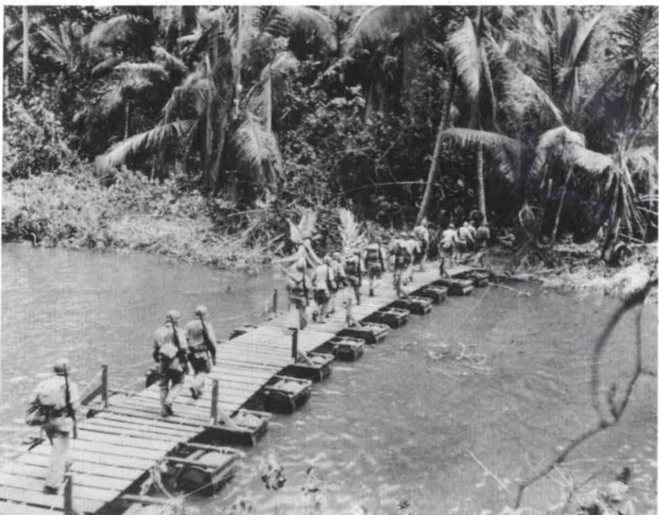
◀ This bridge was one of three constructed by the 1st Engineer Battalion to support the 1 November Marine attack. The bridges were constructed on the night of 31 October. Made out of fuel drum floats and other bridging materials, they were assembled and positioned quickly. The Marines crossing the bridge are part of the reserve force from the 2nd Battalion, 2nd Marine Regiment. (USMC 51337)
