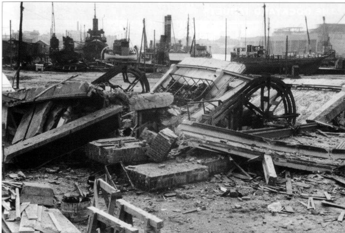
The northern winding shed after Lt Purdon and his demolition team got to work on it. The remains of the great wheels providing the momentum to draw the caisson along its camber can be clearly seen in the centre of the photograph. The background to the picture is the Submarine Basin. (Bundesarchiv, 65/2314A/5A)
