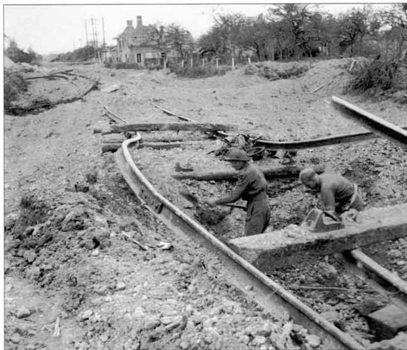
The effects of the heavy bombing raid on Sannerville. The railway line through the village has been torn apart and the whole area was covered with overlapping craters. (IWM B7576)
