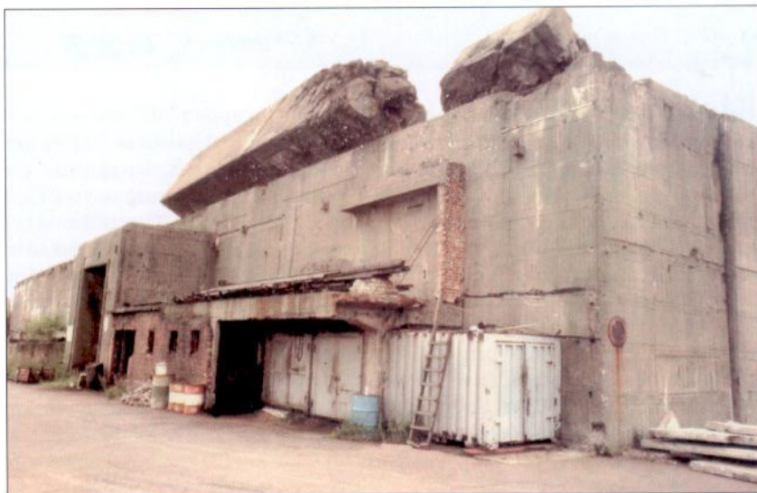
The exterior of the Elbe II bunker. The interior walls were blown out and the roof collapsed: its massive sloping slabs are clearly visible leaning against the top of the remaining wall.
