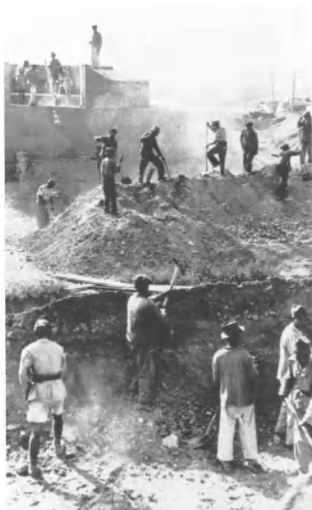
Above: Like ants on an ant heap, this mass of labourers is working on an earthen pile, possibly the basis for a gun position. CIOS Jersey
