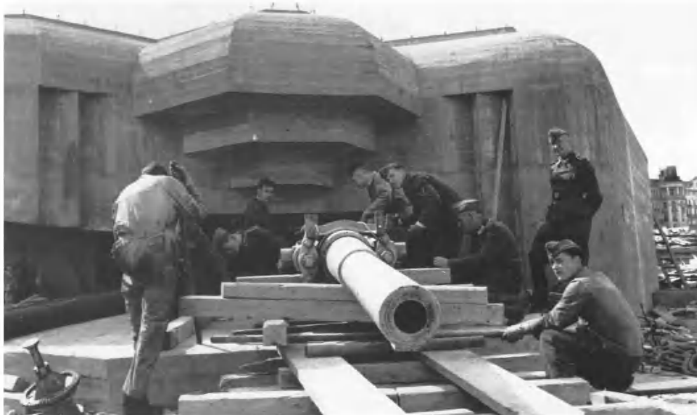
Above: Once the concrete casemates had been built, then the guns had to be installed, such as here, near Ostend, during the summer of 1943. Bundesarchiv
